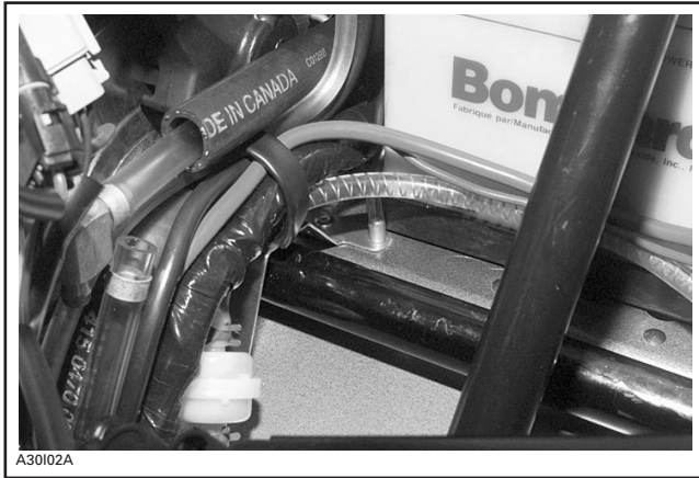
VENT TUBE PROPERLY CONNECTED
